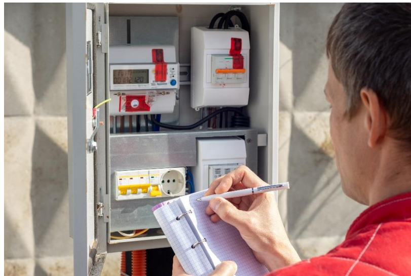
Taking a reading from an electricity meter
